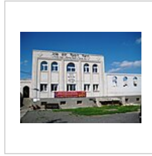
New guesthouse and synagogue next to Ohel of Baal Shem Tov (work in progress); August 4, 2008
